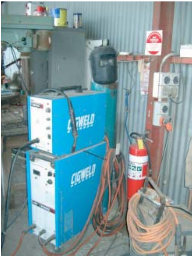
Fire extinguisher readily available
