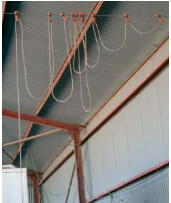
Extension cord suspended off the floor
