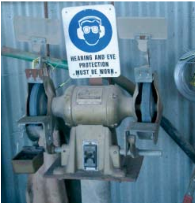
Bench grinder with appropriate guards in place
