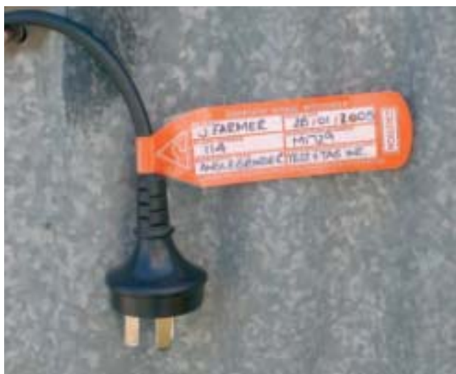
Electrical inspection tag
